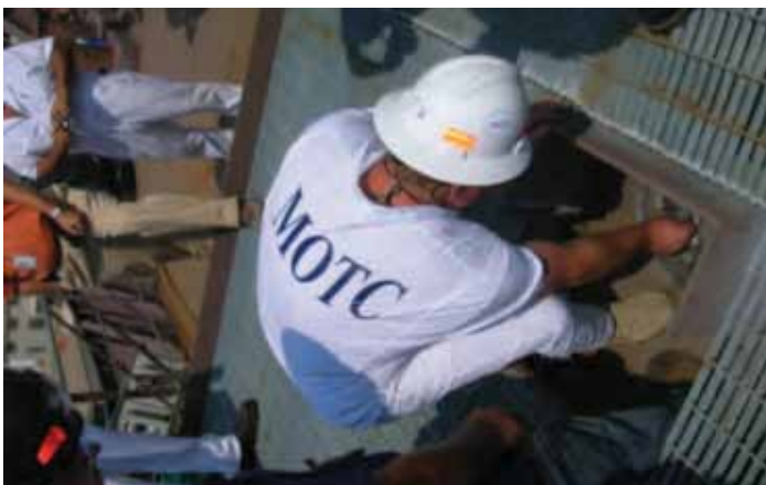
One of the owner's technical reps places the second set of coins under the mast
